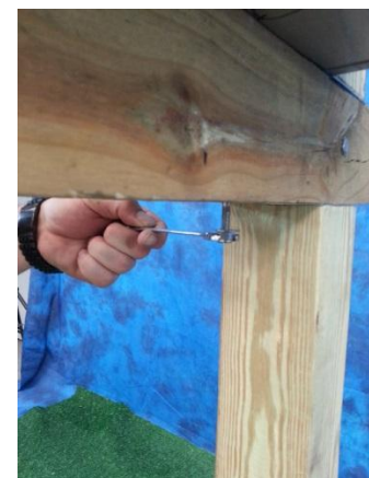
COMPLETE THE INSTALLATION BY TIGHTENING THE LOCK NUTS DOWN WITH A BOX WRENCH
